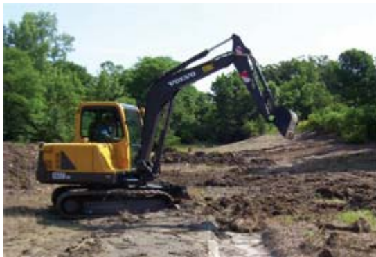
Concrete gutter removal was one aspect of Ohio's first detention basin retrofit.
