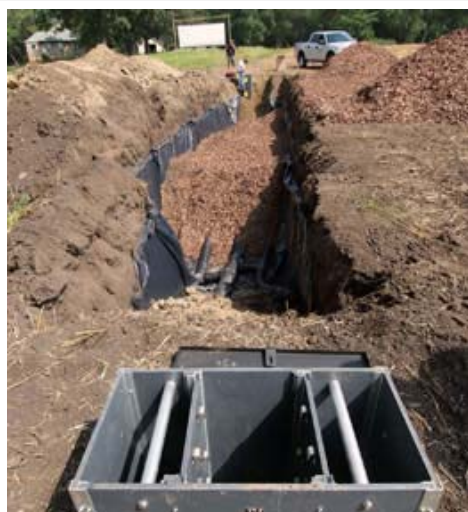
The 80 cubic yards of wood chips in this bioreactor can treat drainage water from 80 acres of Tony Thompson's cropland. Bioreactors have been shown to cut nitrate levels in tile drain water by half.
