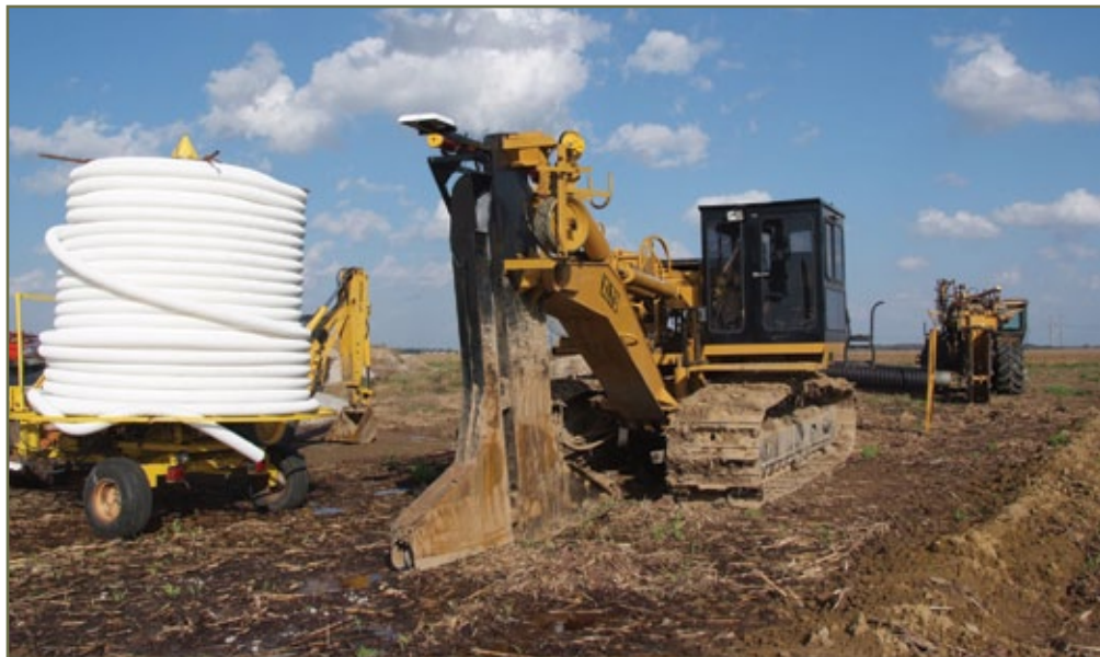
Drainage contractor Rob Wood points out that installing a controlled drainage system requires careful planning before the first foot of tile is laid.
